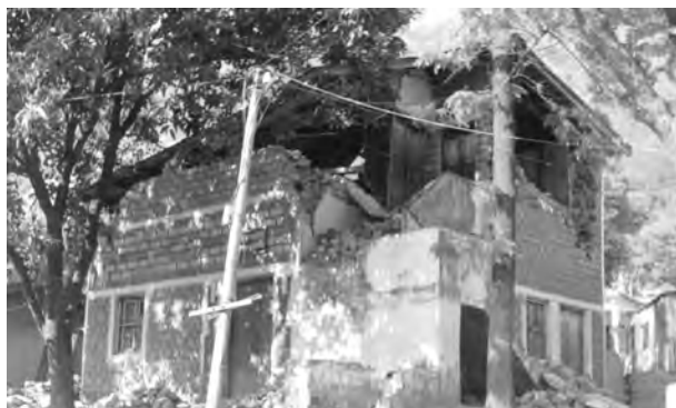
Figure 7.1 : A Damaged Building Due to an Earthquake
